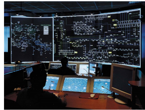
Communication networks Supervisory Control and Data Acquisition (SCADA) system
